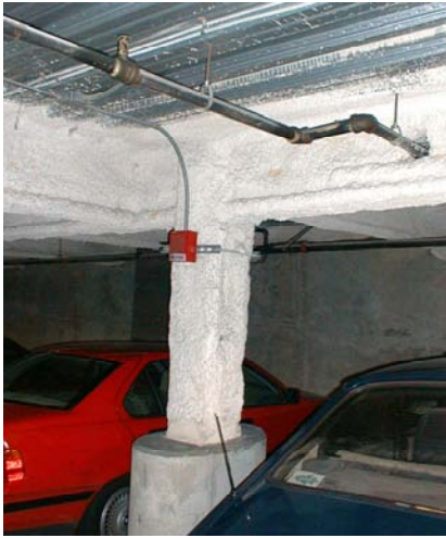
Figure 3-11 Interior view showing fire-proofed columns and beams, which indicate a steel building (S1, S2, or S4).
