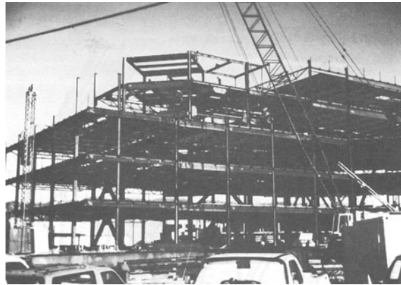
Figure E-13 Braced steel frame, with chevron and diagonal braces. The braces and steel frames are usually covered by finish material after the steel is erected.
