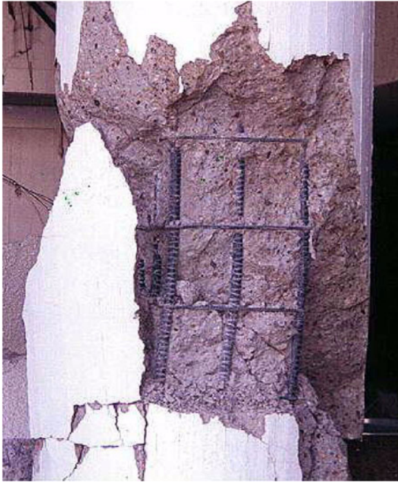
Figure E-27 Example of ductile reinforced concrete column, 1994 Northridge earthquake; horizontal ties would need to be closer for greater demands.
