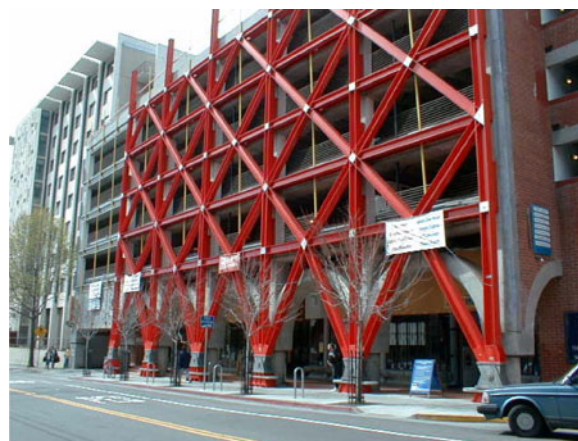
Figure E-15 Rehabilitation of a concrete parking structure using exterior X-braced steel frames.
