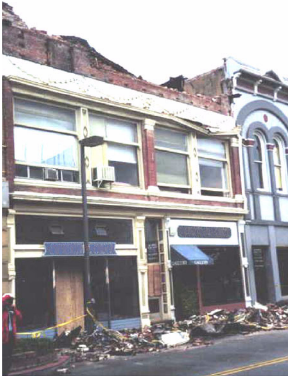
Figure E-53 Parapet failure leaving an uneven roof line, due to inadequate anchorage, 1989 Loma Prieta earthquake.
