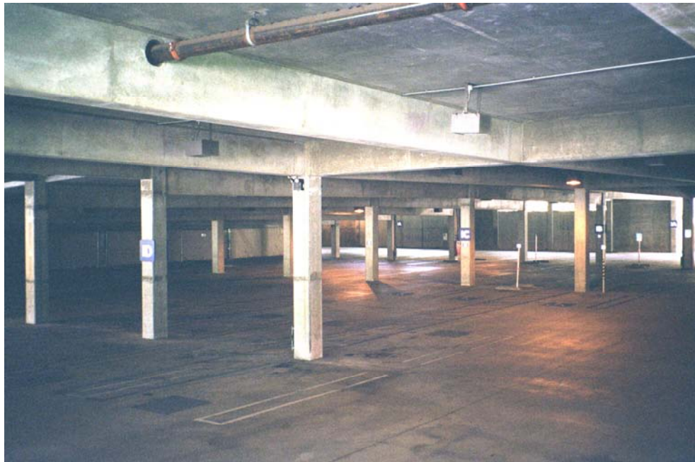
Figure 3-12 Interior view showing concrete columns and girders, which indicate a concrete moment frame (C1).
