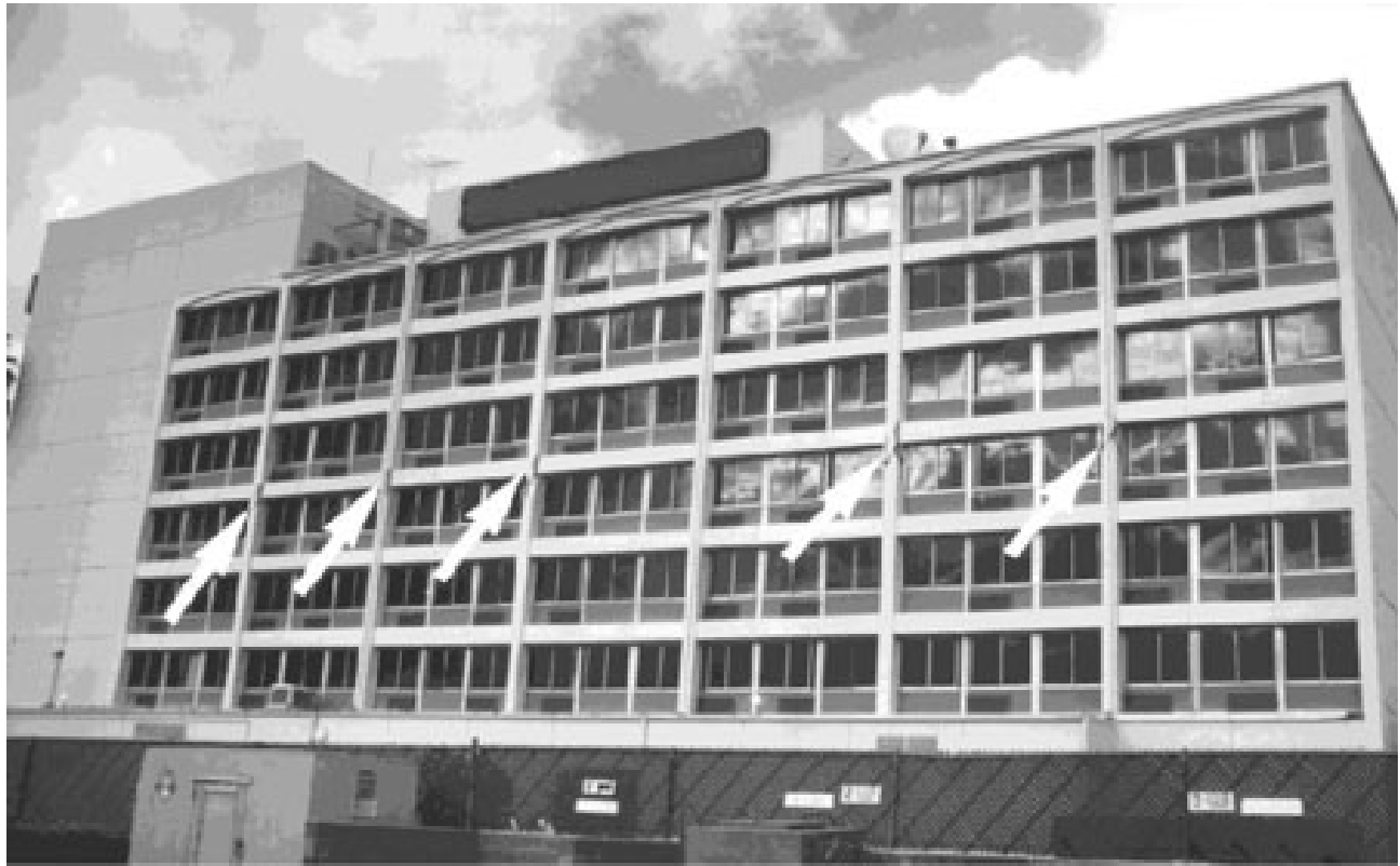
Figure E-29 Locations of failures at beam-to-column joints in nonductile frames, 1994 Northridge earthquake.
