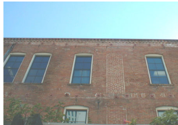
Figure E-55 Upper: Two existing anchors above three new wall anchors at floor line using decorative washer plates. Lower: Rehabilitation techniques include closely spaced anchors at floor and roof levels.
