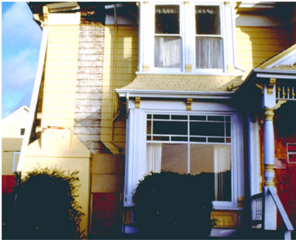
Figure E-9 Failure of post and pier foundation, Humboldt County.
