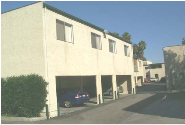
Figure 3-16 Example of soft story conditions, where parking requirements result in large weak openings.
