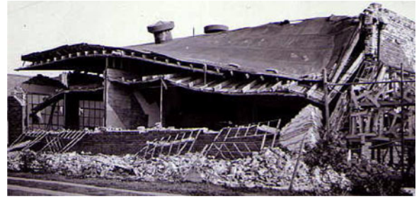
Figure F-11 Collapse of unreinforced masonry bearing wall, 1933 Long Beach earthquake.
